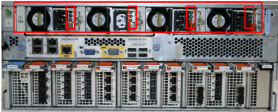
Figure 147. Four power supplies
